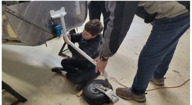
Jude Murphy bolting on the new nose gear leg as part of SB19-08-26 upgrade.
