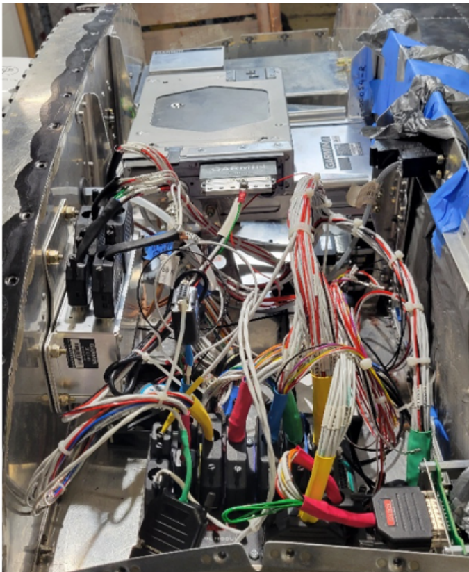
Photo of avionics and wiring harness. Some organization of routing and final connections are still required.
